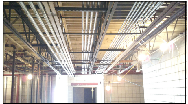
Photos above: Exterior and interior views of the ND National Guard Readiness Center under construction at Camp Grafton.
